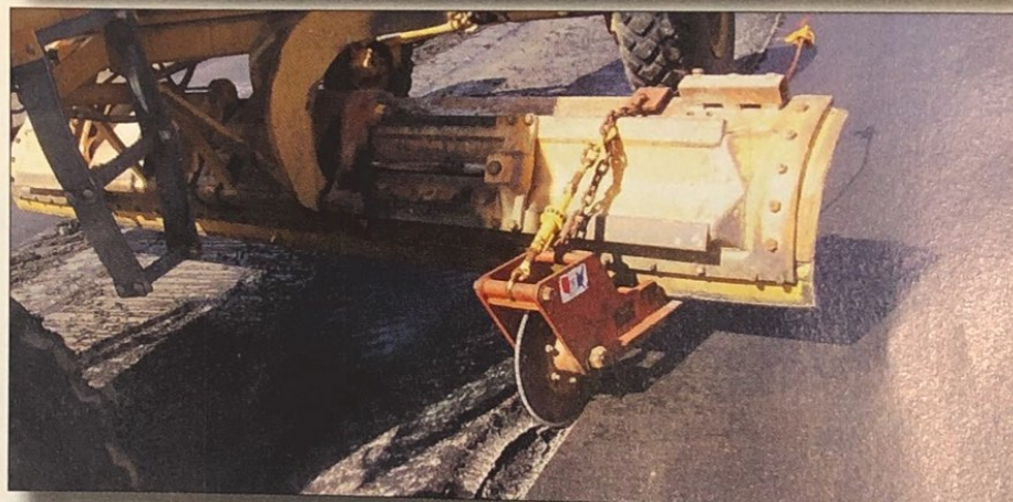
The track was paved top down, placing the unconfined edge of the longitudinal joint on the downhill side. The unconfined edges were cut back using a cutting wheel mounted on a motor grader while the pavement was still plastic.
