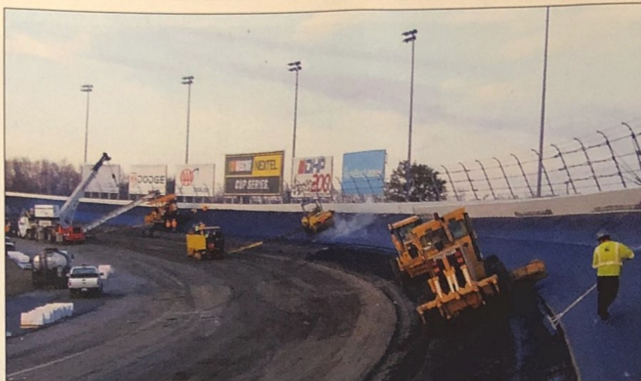
Although the average mill depth was 3.5 in., the actual depth was adjusted throughout the track to remove age-induced bumps. In the turns, a hydraulic stiff-arm, connected to a bulldozer, supported the mill.
