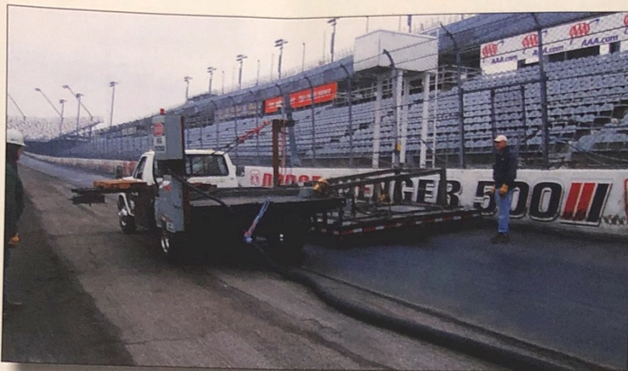
Here a surface heater is used to dry the pavement and break tack. Lane combined an old truck and a number of infrared heaters to do the job.
