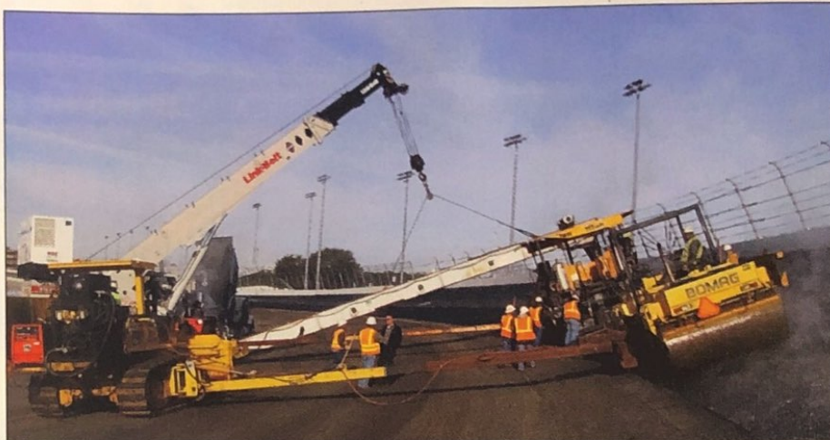
Tandem end-dump trucks dumped into a Roadtec material transfer vehicle, which in turn fed a hopper on a crane-mounted slat conveyor and finally loaded a hopper insert on the Ingersoll Rand Titan ABG-525 paver.
